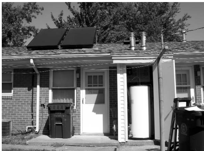
Solar water heaters and collection tank at the Housing Authority of Owensboro
